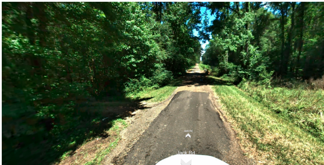
Uneven pavement on the project section. Also note that the existing road is too narrow for two vehicles to pass.
